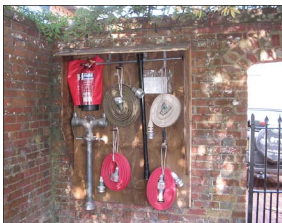
Figure 18: Provision of firefighting equipment
